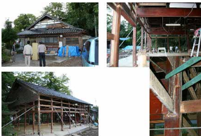
◀ Image Ref. 3.72 Example of restoration work undertaken using traditional techniques Source: Yasumichi Murakami
